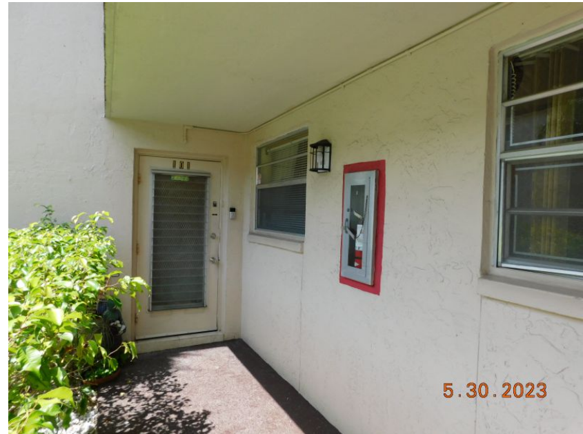
Unprotected Window and Unprotected Glazed Entry Door
