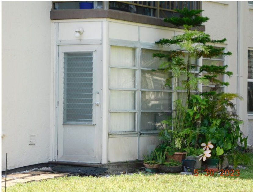
Unprotected Window and Unprotected Glazed Entry Door
