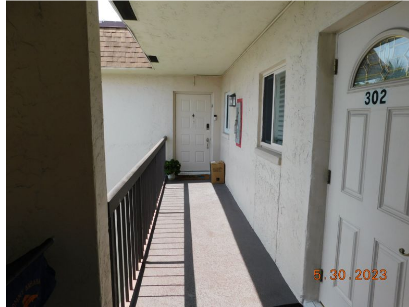
Unprotected Solid Entry Door
