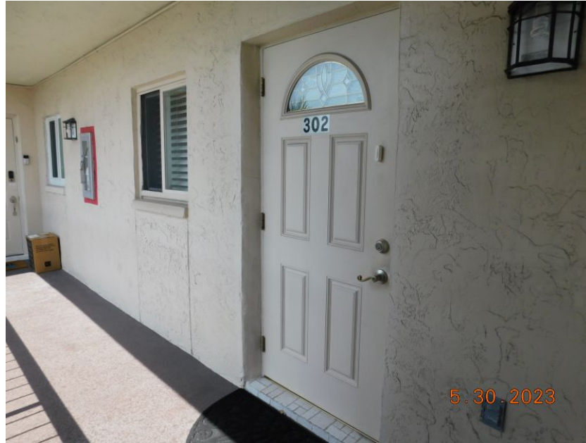
Unprotected Window and Unprotected Glazed Entry Door
